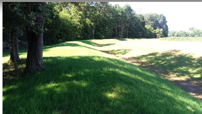
Grade Stabilization Structure constructed by B&D Siteworks at Ryan Farm in Leonardtown
